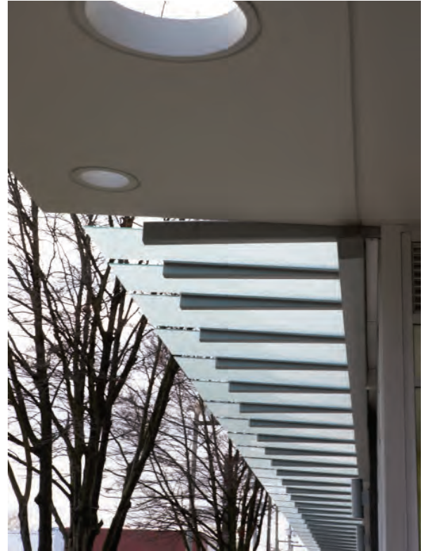
Example of a continuous weather protection option, such as along exterior building walls directly adjacent to pedestrian networks and areas (guideline 59).
